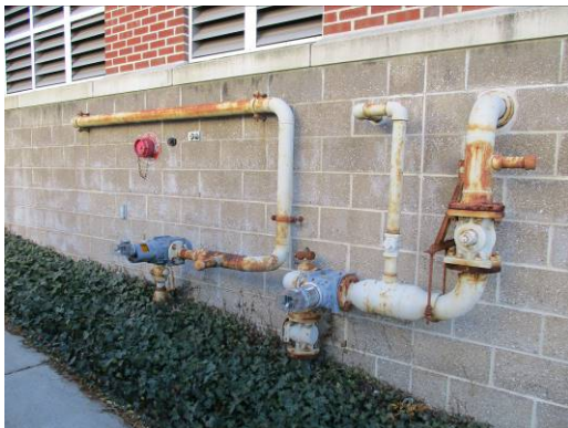
Gas services and meters
