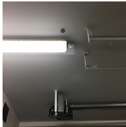
Wall type Sensor on Ceiling in Sallyport
