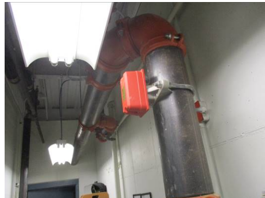
Main Building flow switch
