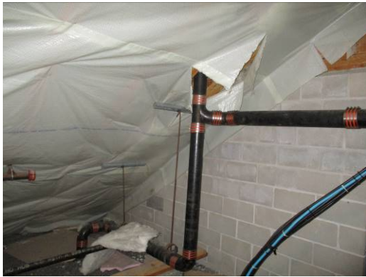
Cast iron vent piping in attic
