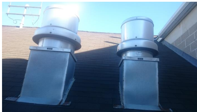
Typical Exhaust Fan
