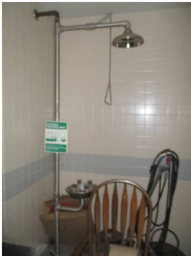
EMT Washroom emergency fixture
