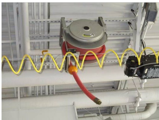
Apparatus Bay typical fill valve
