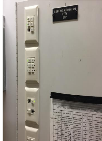
Lighting Relay Panel
