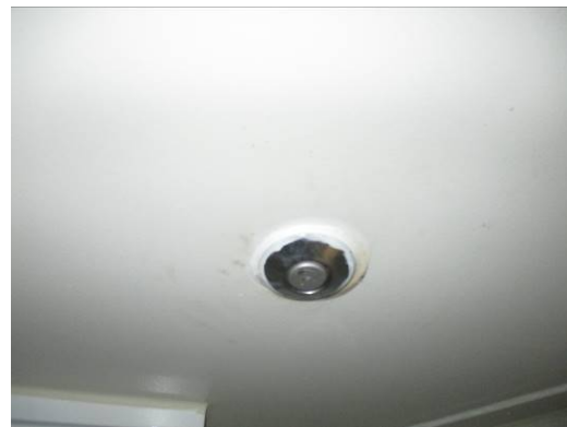
Typical institutional type sprinkler (in cell)
