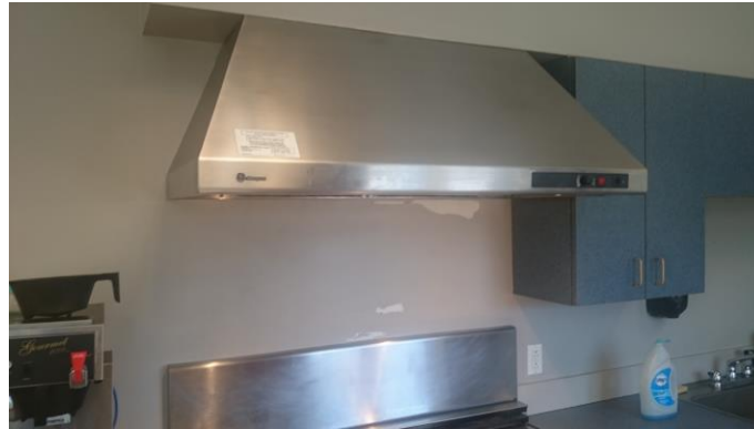
Fire Station Kitchen Hood
