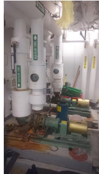
Chilled Water Pumps
