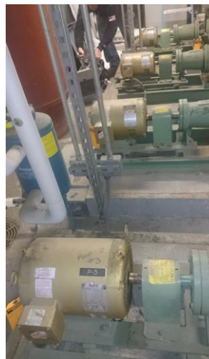
Base Mounted Pumps
