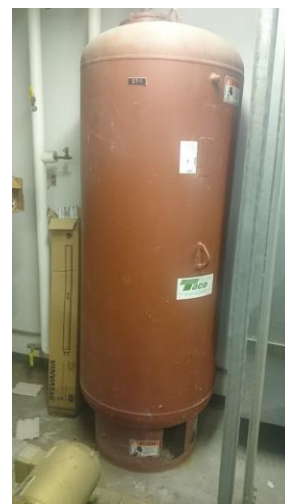
Expansion tank & Air Combustion
