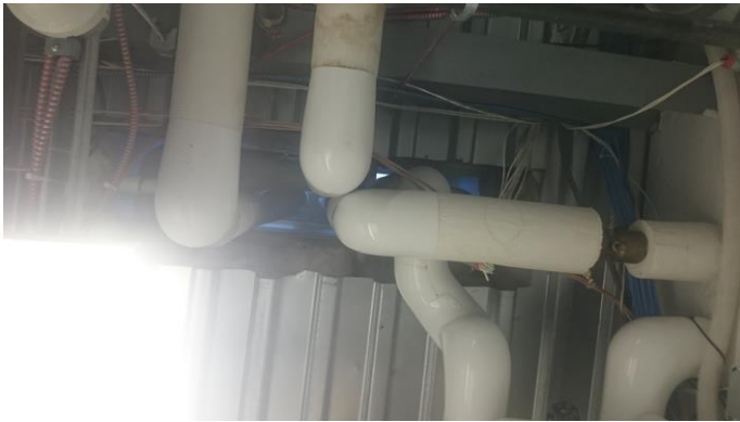
Pipe Mains to RTU-2
