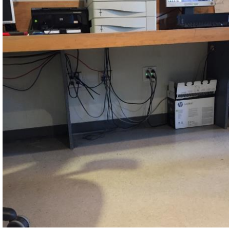
Fire Dept. Dispatch Console
