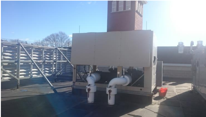
Roof Mounted Chiller
