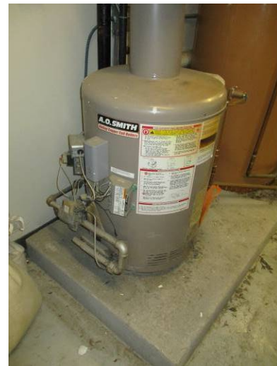
Domestic water heater
