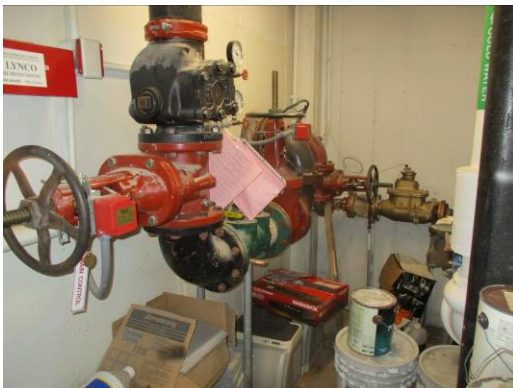
Building fire service entrance
