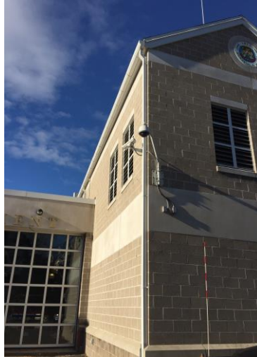
CCTV Camera Exterior
