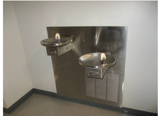
Electric water cooler
