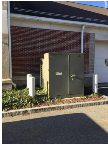
Pad Mounted Transformer
