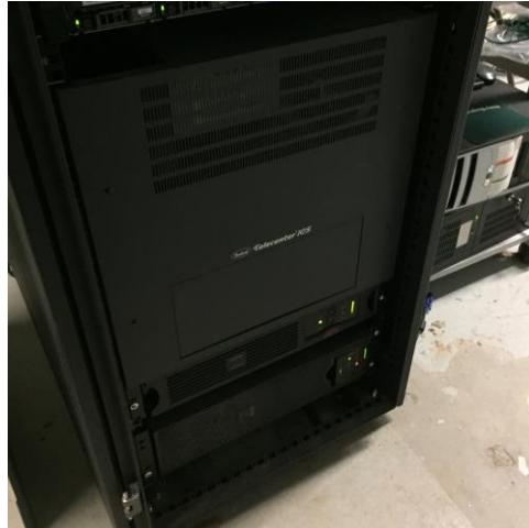
Paging System in Telephone Room
