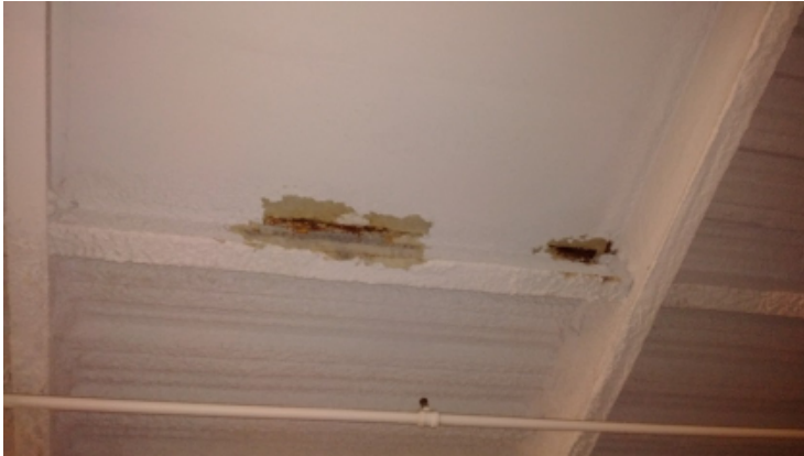
Photo 2, Rebar Corrosion in Concrete Deck
