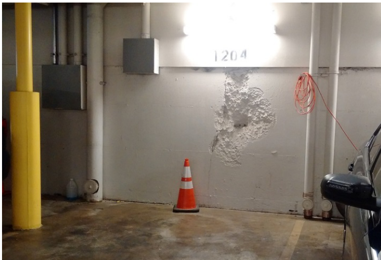
Photo 1, Damaged Concrete Wall
