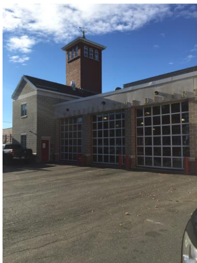
Building Wall Packs
