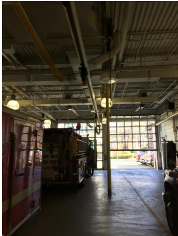
Apparatus Bay Lighting
