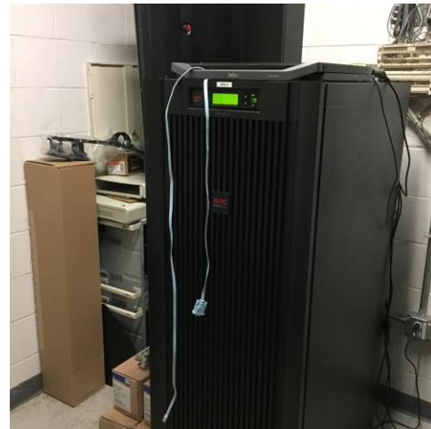
UPS in MDF Room
