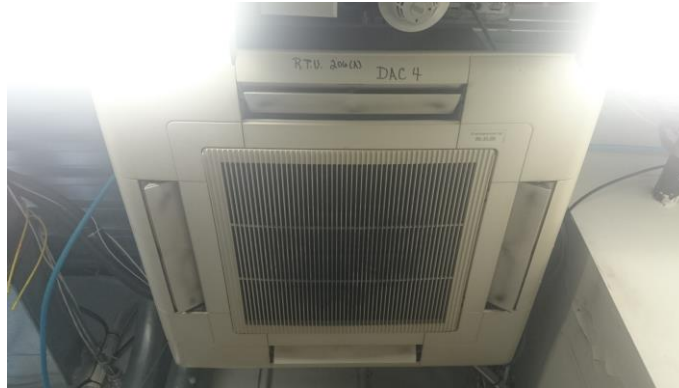
Ductless Cooling units
