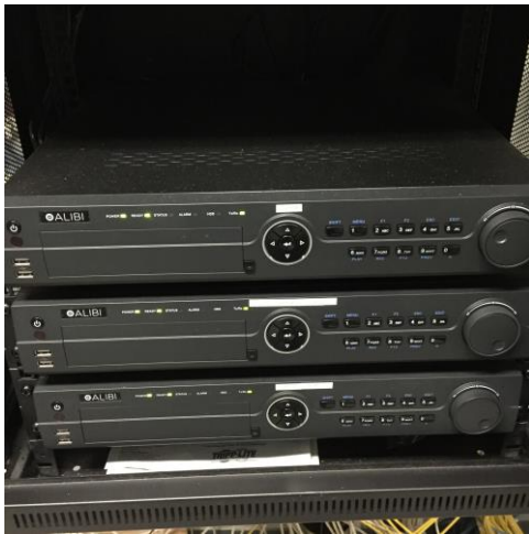
CCTV Camera Exterior NVRs
