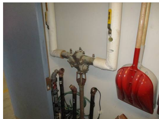
Reduced pressure backflow preventer – App Bay
