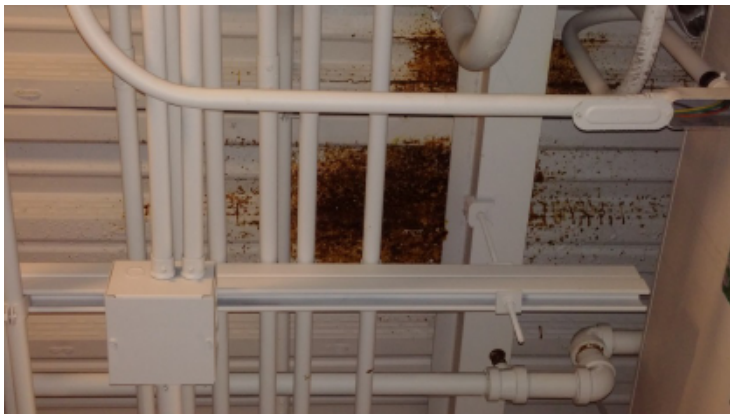
Photo 3, Rusted Metal Deck
