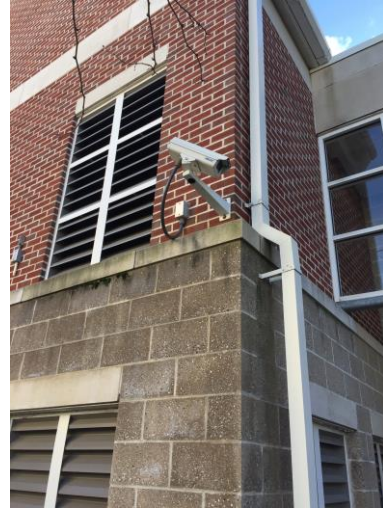
CCTV Camera Exterior
