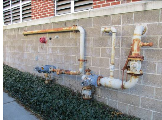
Fire Department connection
