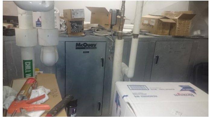
Air Handling Unit
