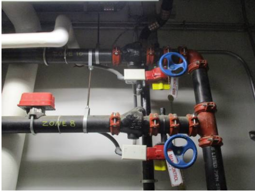
Typical sprinkler zone control valve assembly
