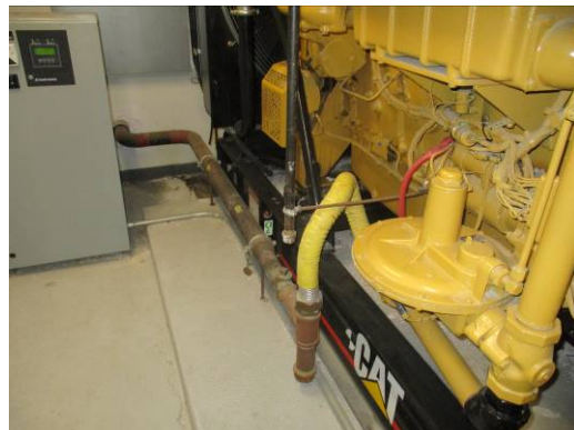
Gas supply to generator
